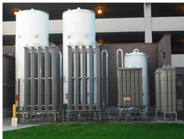
Figure 9. A typical hospital liquid oxygen system. There are 2 main liquid vessels and 1 reserve smaller vessel to the right. The evaporating coils, where liquid oxygen is converted to gas are in the foreground and in this figure have no ice accumulation.
