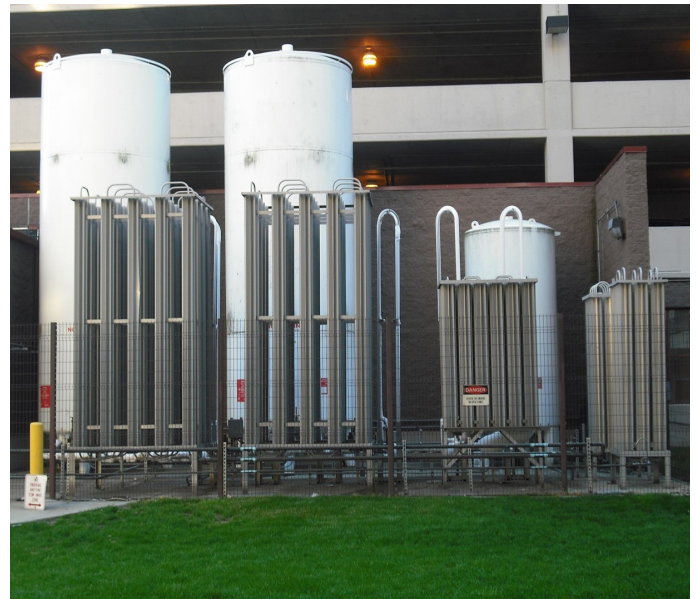
Typical hospital liquid oxygen system including two main reservoirs and a smaller reserve reservoir. The vaporizing coils are in the foreground.
